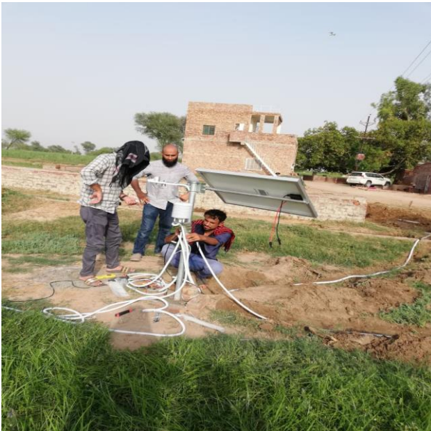
IWMI team troubleshooting a solar pump in the Jhang district.
