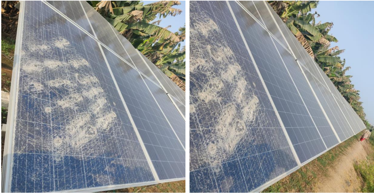
Fig 1: Panels got damaged by a mischief person in NAVAPARA feeder in DGVC
