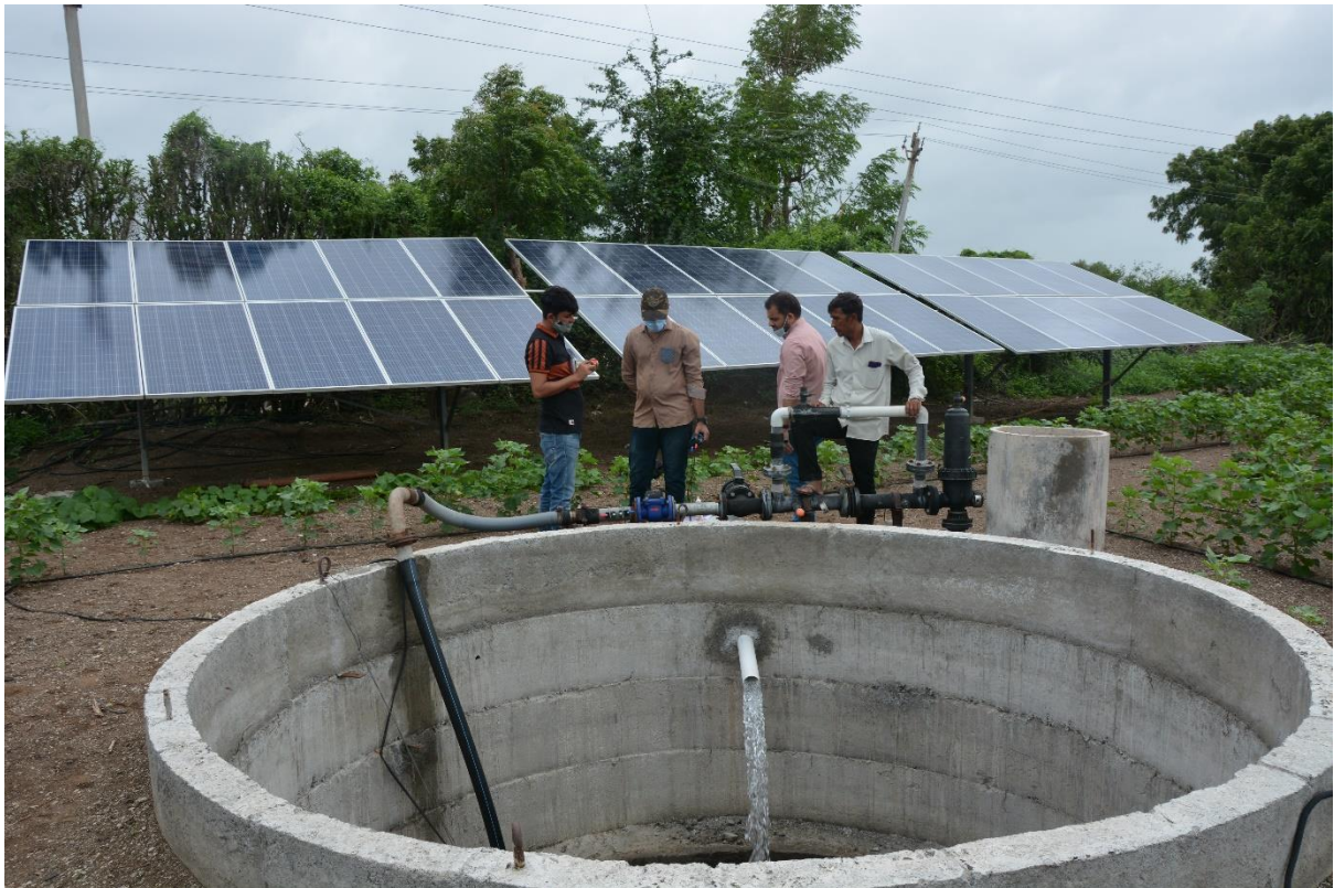
Picture 3: Picture showing solar panels and a dug well from Parameshwar feeder in Botad district, Gujarat Photo: Yashodha Yashodha/IWMI
