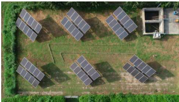
A solar irrigation pump site at National Agricultural Research Centre (NARC) Chak Shahzad Islamabad, Pakistan (photo: IWMI Pakistan).
