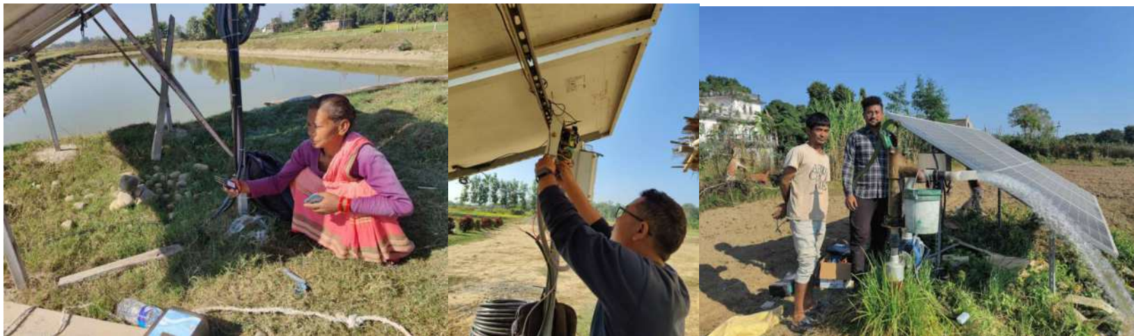
Figure 22: Reinstallation of Gham Power Krishi Meter (Upgraded) version in the SWPS installation site of AEPC and Gham Power
