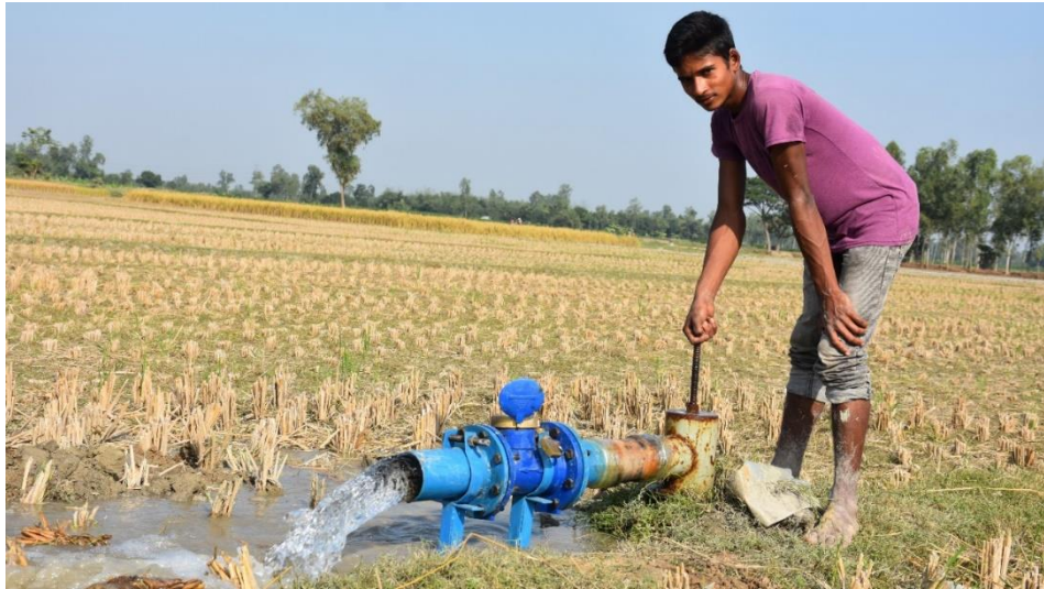
Installed flow meters at a water outlet in solar irrigation command area Photo: Via NGO Forum
