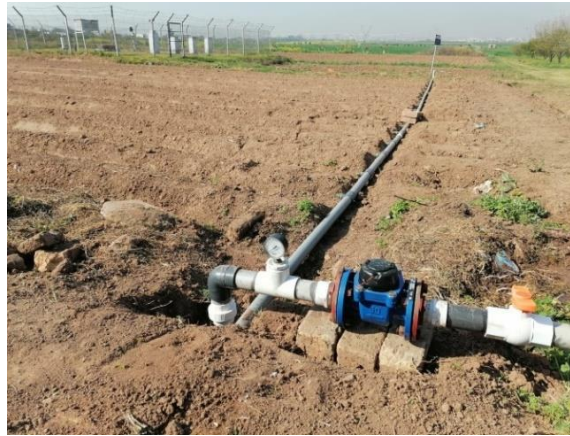
Picture 3: Water meter and pressure gauge
